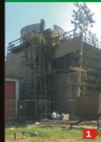
1 Original Crossflow Tower
